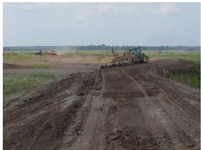
Figure 13–25 Dike for internal water control
