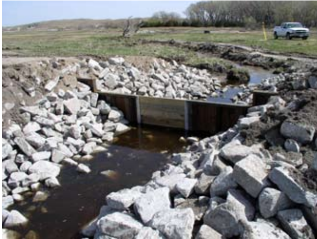
Figure 13–32 Sheet pile weir with stoplogs
