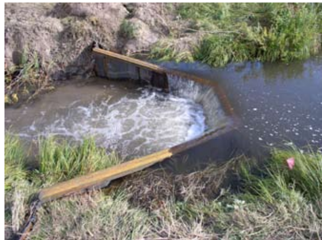
Figure 13–31 Sheet pile vortex weir
